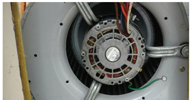
A clean furnace blower protected for years by an Aprilaire air purifier.
