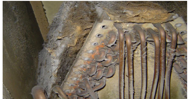
A dirty and frozen AC coil caused by a sub-par one-inch filter and an irregular filter replacement schedule.
