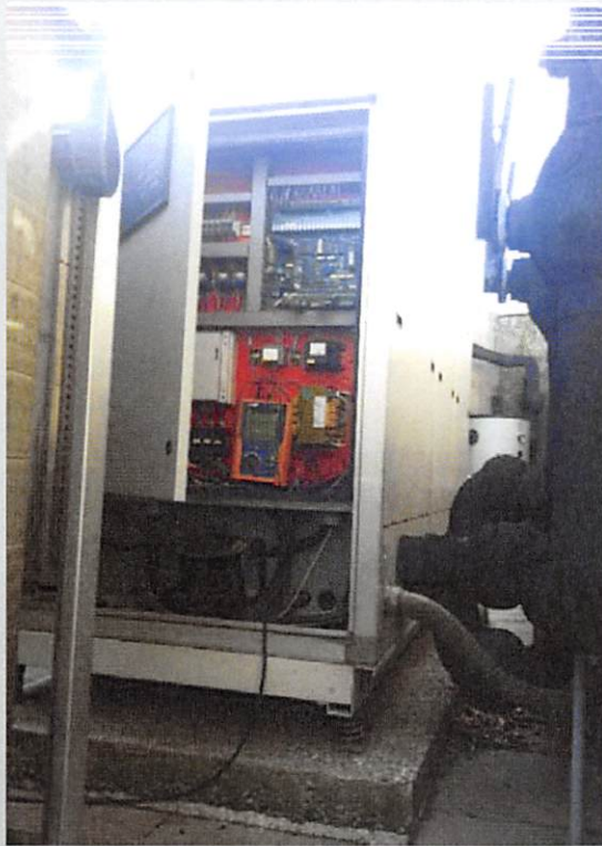
Cooling unit with network analyser
