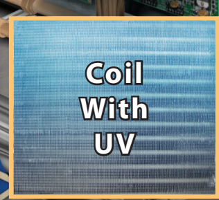
UV-C light suppresses microbial growth on HVAC coils and surrounding areas
